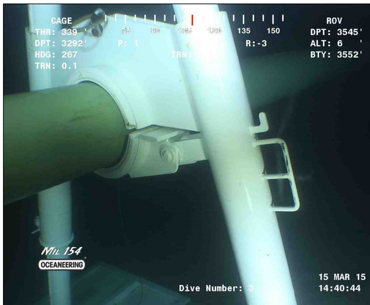
16 In. Pipeline Pipe Span Supports
