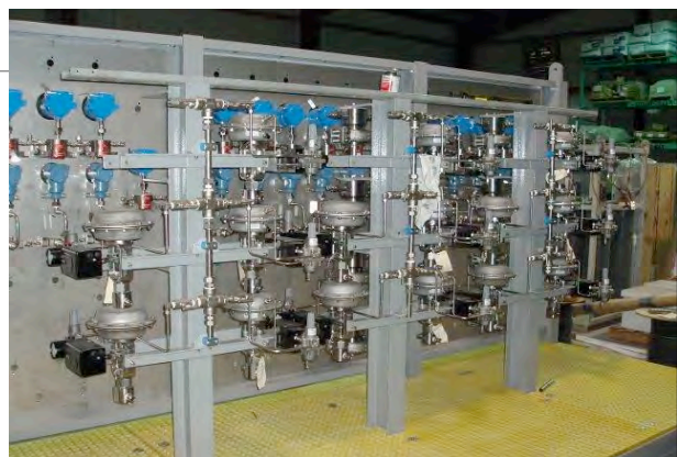
Methanol Distribution Skid
