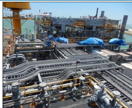
Topsides View of Delta House FPS
