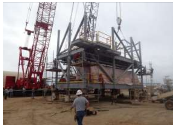
Setting Second Level of Chemical Injection Module
