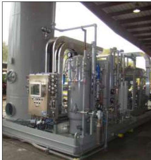
Instrument Air Skid
