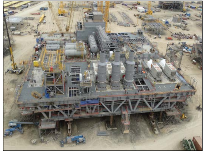
Delta House Topside
