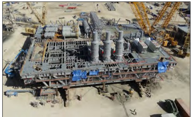
Delta House Topside
