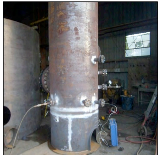
1st Stage Scrubber
