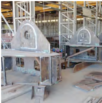
2/14—Four pad eye node sections in progress in the structural assembly building
