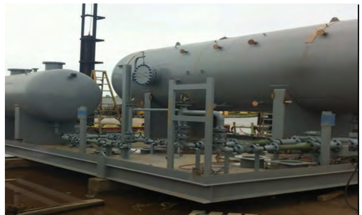
Overall Flare Scrubber Skid to this point
