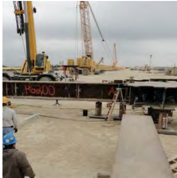
2/20—Fitting the first plate girder to the center node section on the lower level pancake
