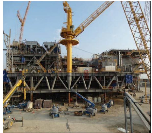
Delta House Topside
